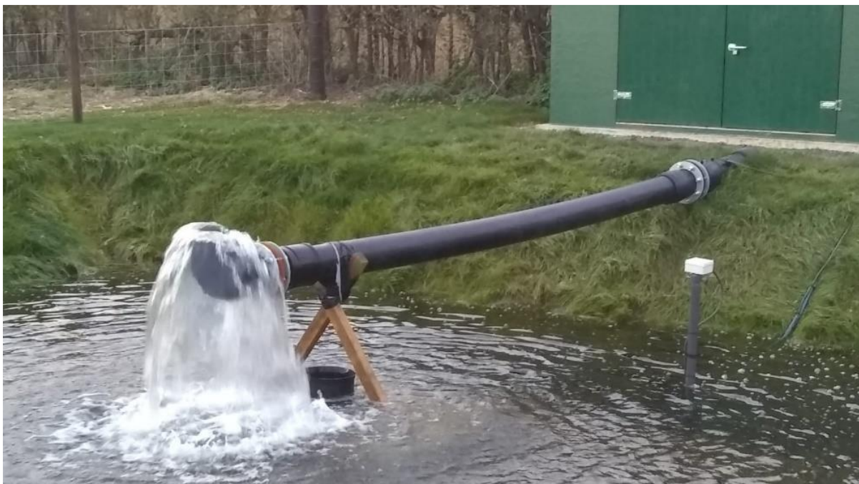
Figure 5. Photograph of recharge lagoon in operation
